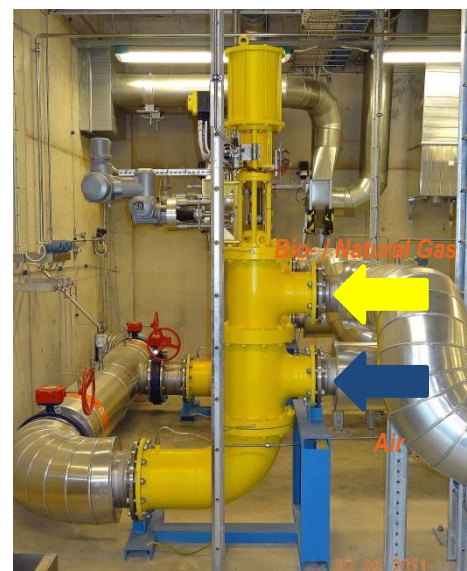
Figure 5 Two Dimensional Gas Mixing Valve installed in Main Conditioning / Feeding Unit
